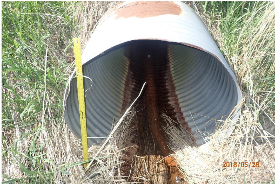
Reach UCT1 flows into a CSP at Brock Street at the downstream extent of the property. Iron staining was noted at the downstream extent, but no where else in the reach.
