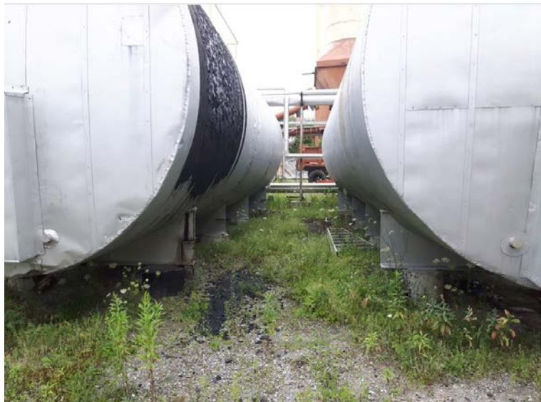
Photo 8 – View of two asphalt cement storage tanks.
