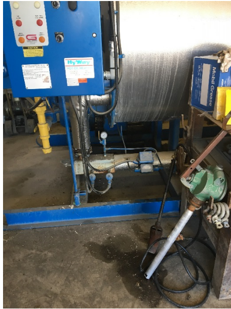
Photo 11 – View of minor staining on floor of boiler house.
