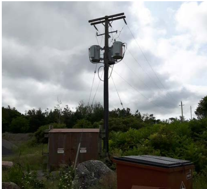
Photo 6 – View of a transformer present south of the asphalt plant.
