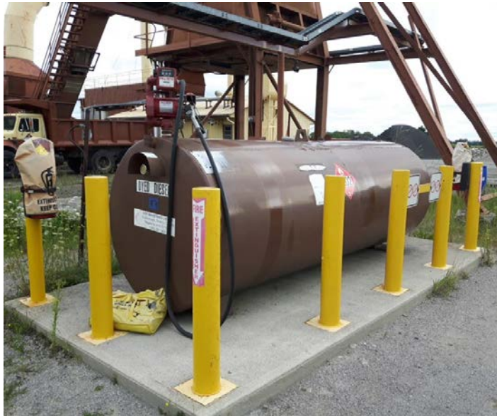
Photo 3 – View of a 4.540 L diesel AST.
