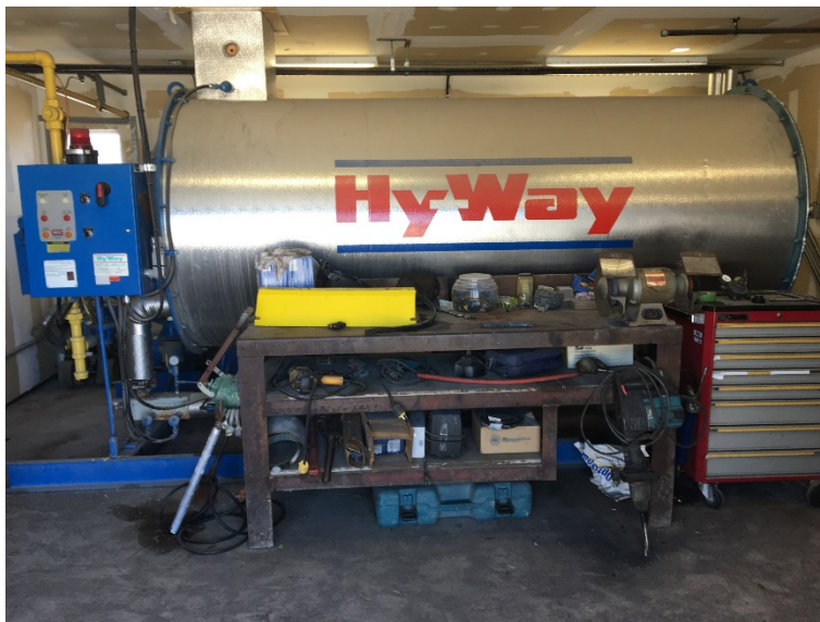
Photo 12 – View of liquid asphalt heating boiler.
