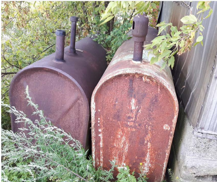
Photo 10 – Fuel oil ASTs present in the yard on the east side of the house at 4529 Concession Road 7.
