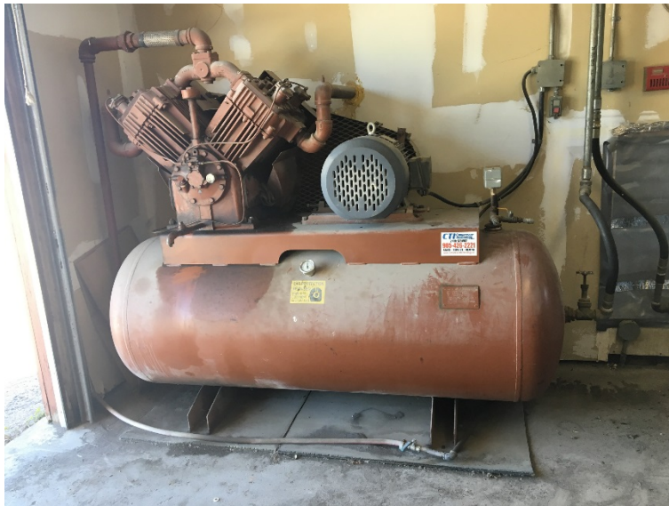
Photo 14 – Air compressor in boiler house.
