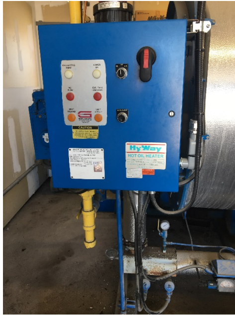
Photo 13 – View of control panel of the hot oil heater in the boiler house.
