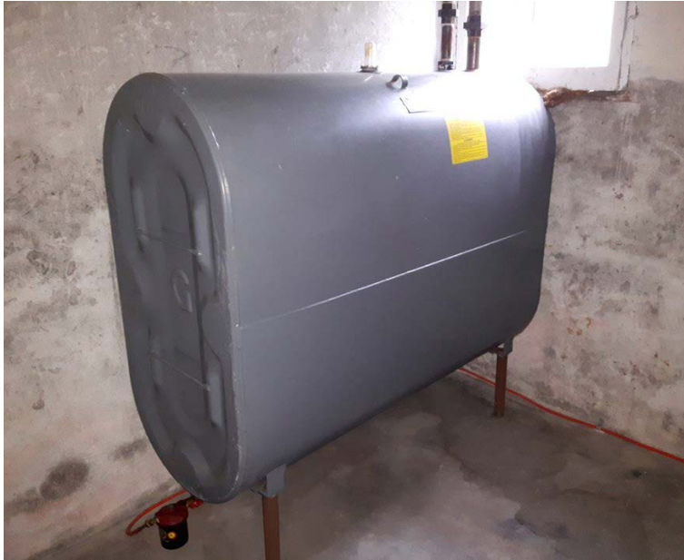
Photo 9 – View of fuel oil AST in the basement of the house at 4589 Concession Rd 7.
