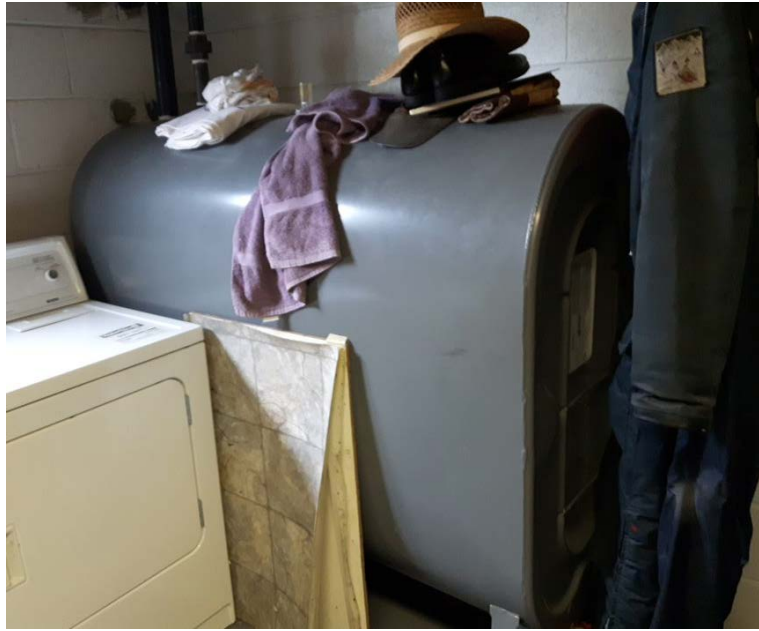
Photo 7 – View of fuel oil AST in the basement at 4499 Concession Road 7.
