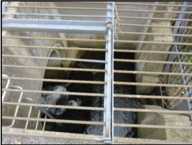
Photograph 1. Reach UBT-1 Outlet structure of existing upstream online pond, south of Bolton Drive.
