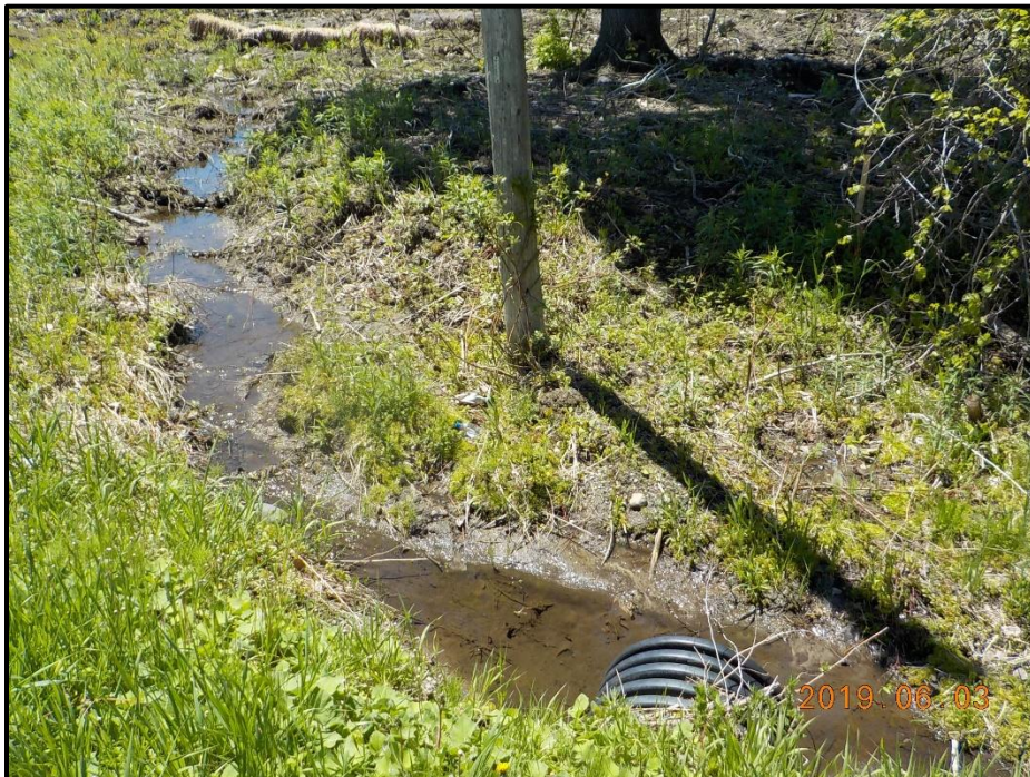
Photograph 8. Condition of HDF 4 on June 3, 2019
