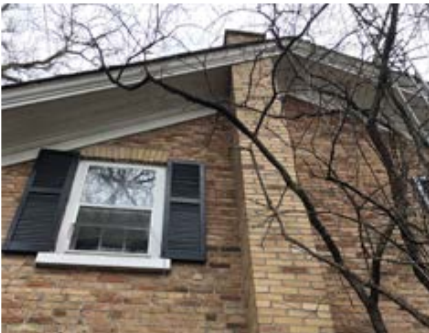
Figure. 3.30. Incompatible existing chimney is not original and is to be removed
