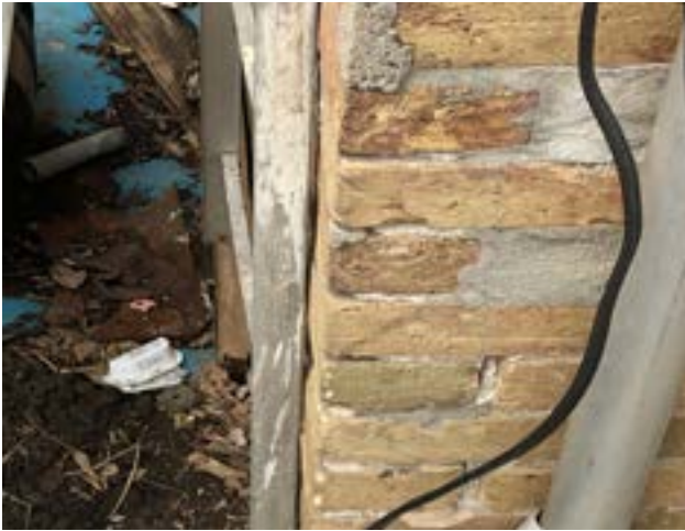
Figure. 2.12. Southeast corner brick & mortar in fair condition; missing brick
