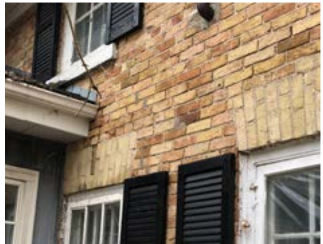
Figure. 2.20. West facade: Facade soiling & missing brick at soldier course
