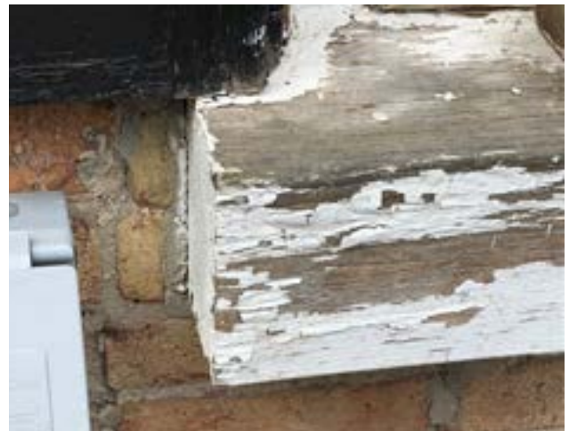
Figure. 3.38. All original windows to be fully restored & sills to be replaced
