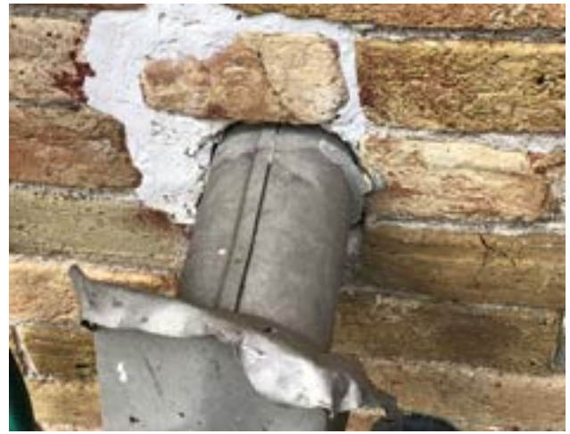
Figure. 2.7. Partially missing bricks and incompatible sealant
