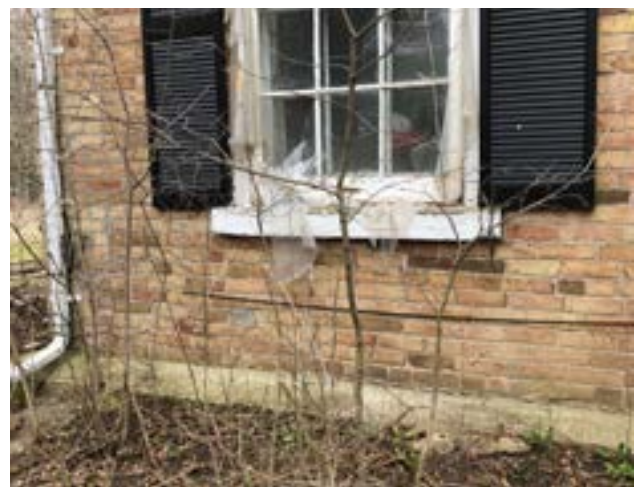
Figure. 2.21. West facade: Soiled & stained brick
