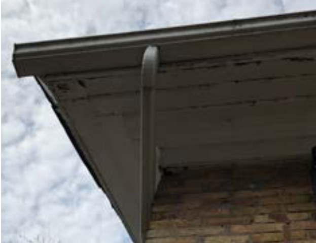
Figure. 2.32. Deteriorated original soffits and fascia
