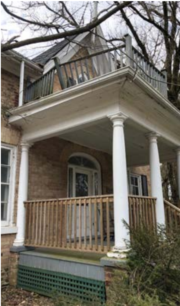
Figure. 3.35. Second floor deck rail to be removed & replaced
