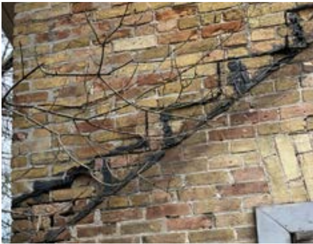
Figure. 2.16. South Facade: Staining & tar from a previously removed shed addition
