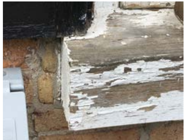
Figure. 2.40. Original lower sills in poor condition
