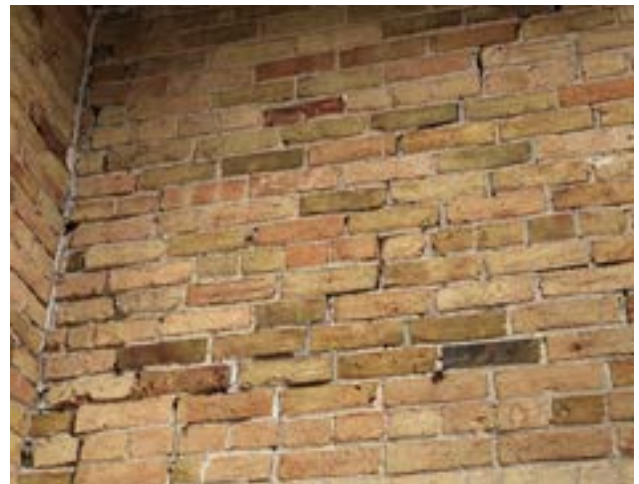
Figure. 2.30. Inner south east corner: brick in poor condition with signs of cracks and open mortar joints
