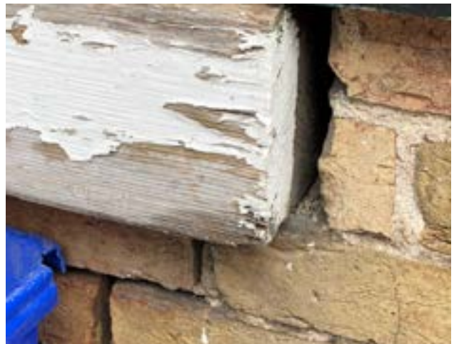
Figure. 2.2. Loose and open mortar joints
