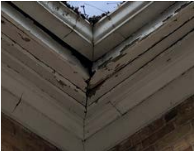
Figure. 3.29. Original wood fascia to be replaced or repaired & repainted
