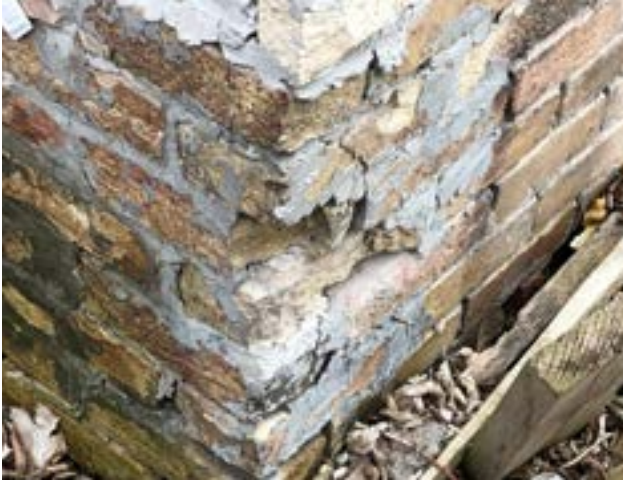
Figure. 2.11. Southwest quoining in poor condition
