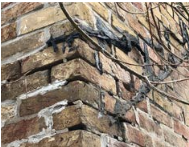
Figure. 2.18. South Facade: Open mortar joints at corner
