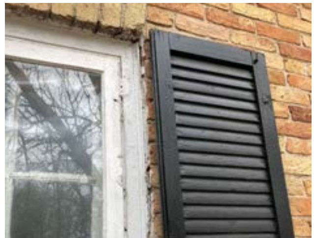
Figure. 3.39. Shutters are not original and are to be removed; brick replaced; mortar repointed
