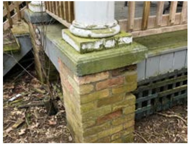
Figure. 3.32. Cracked original brick & wood column bases to be replaced
