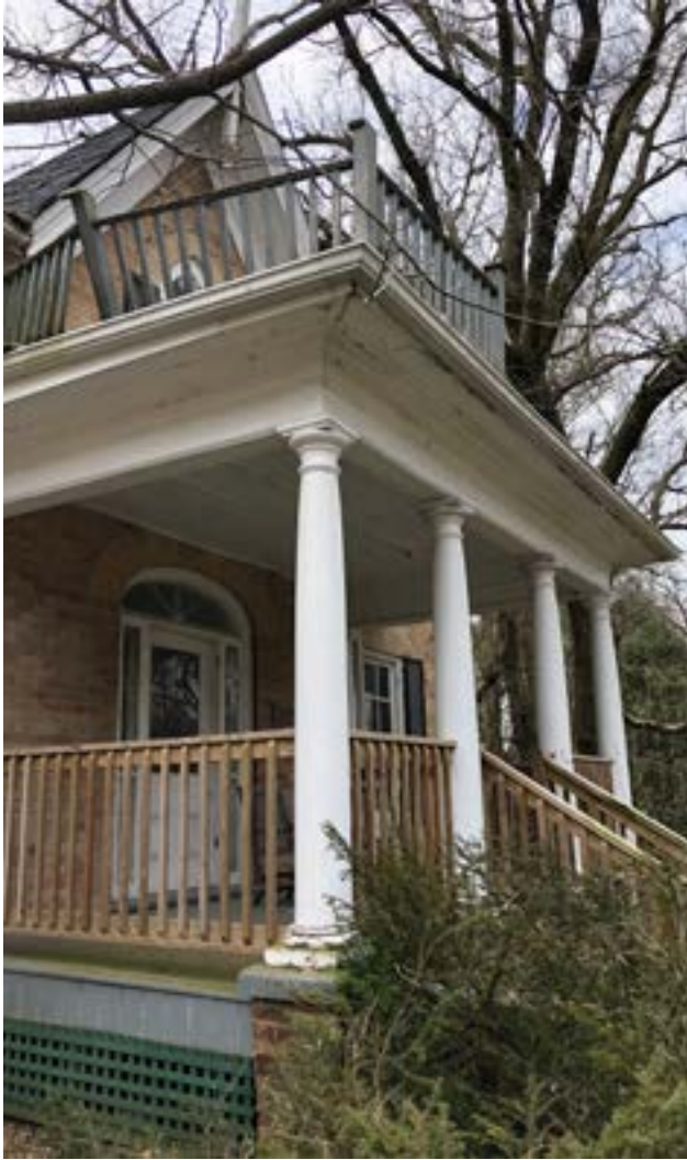
Figure. 2.35. Deteriorated porch railing, deck & skirting
