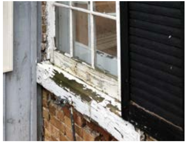
Figure. 2.39. Original lower sills in poor condition
