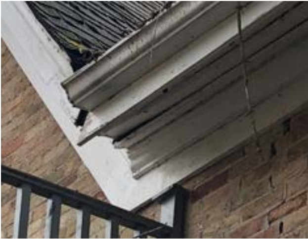
Figure. 2.33. Deteriorated original soffits and fascia
