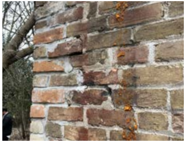
Figure. 2.1. Loose and open mortar joints
