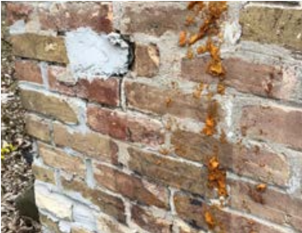
Figure. 3.18. Incompatible mortar to be removed
