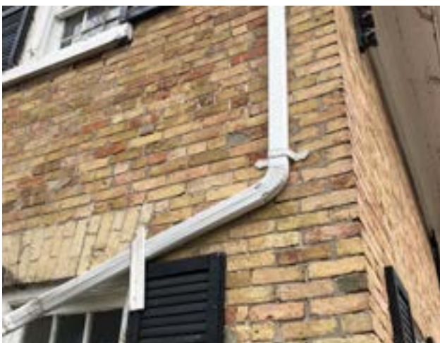
Figure. 3.25. Eavestroughs and downspouts to be replaced
