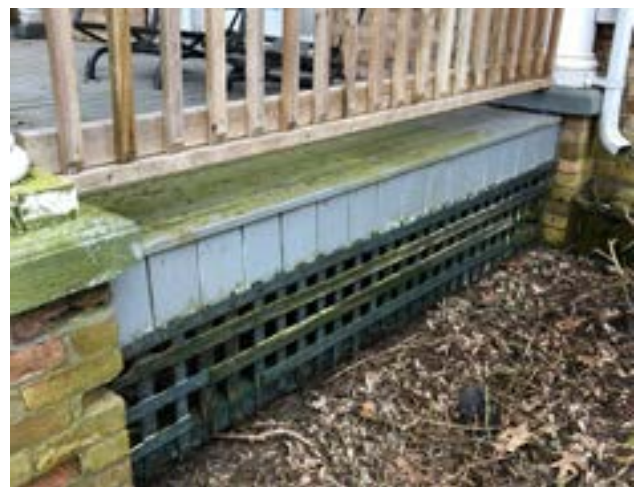
Figure. 3.34. Porch railing, deck & skirting to be removed & replaced
