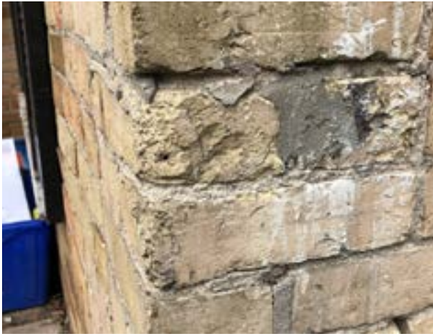
Figure. 2.14. Southeast corner: brick in poor condition
