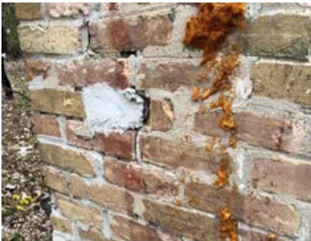
Figure. 2.17. Lower part of southwest corner in poor condition
