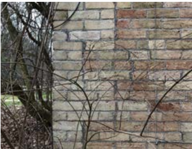
Figure. 2.26. North facade: Staining & environmental soiling
