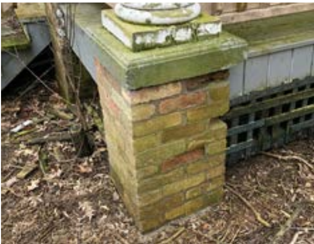
Figure. 2.25. North facade: Missing bricks
