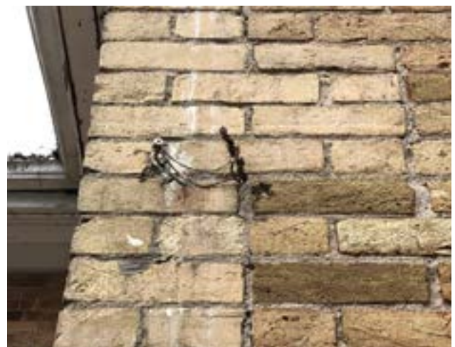
Figure. 2.9. Residual fasteners & penetrations, chipped bricks at the corner
