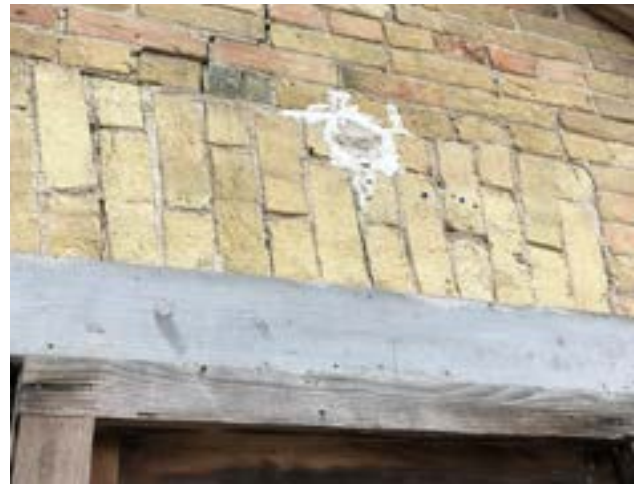
Figure. 2.19. South Facade : Missing bricks & cracks at soldier course above door
