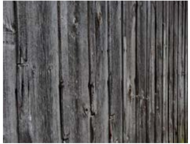
Figure. 3.4. Typical condition of wood at existing driveshed
