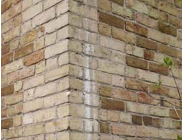
Figure. 2.15. Non-original quoining is in poor condition
