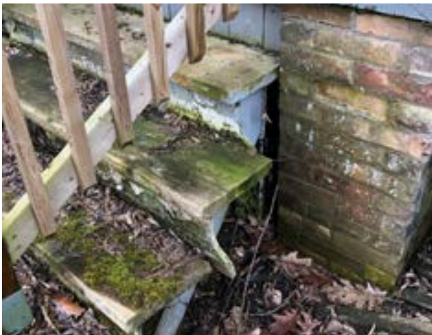
Figure. 2.37. Deteriorated front porch stairs
