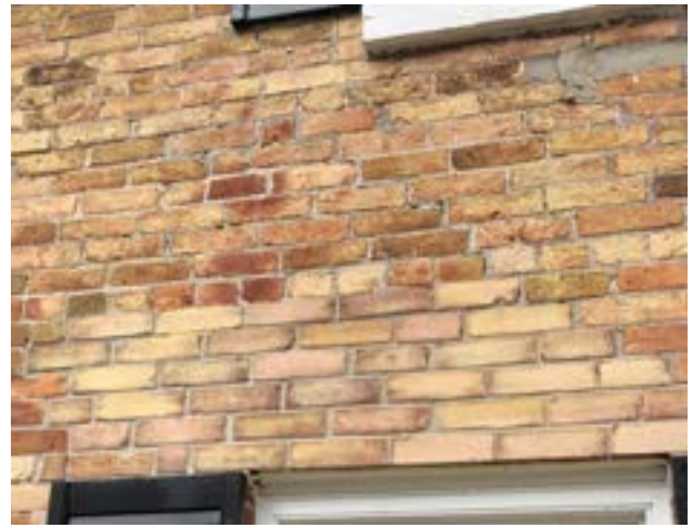
Figure. 2.29. East facade: Incompatible brick from previous repairs
