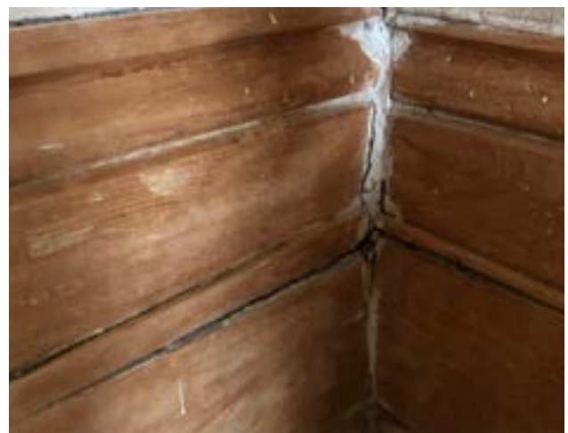
Figure. 3.44. Original baseboards to be preserved, repaired & repainted
