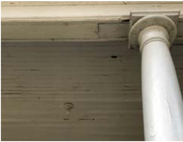
Figure. 2.34. Deteriorated original soffits and fascia
