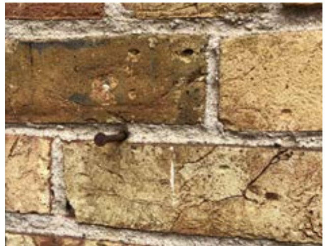
Figure. 3.27. Detail of extraneous items to be removed
