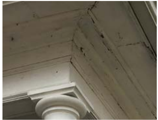
Figure. 3.37. All original wood elements at porch to be repaired and repainted
