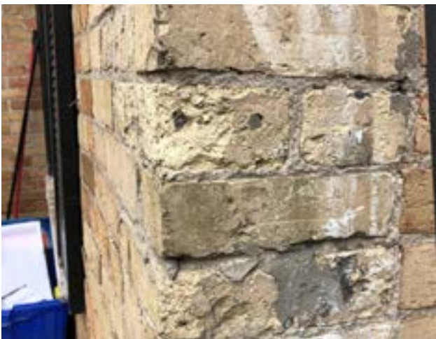
Figure. 3.19. Spalled & cracked brick to be removed & replaced
