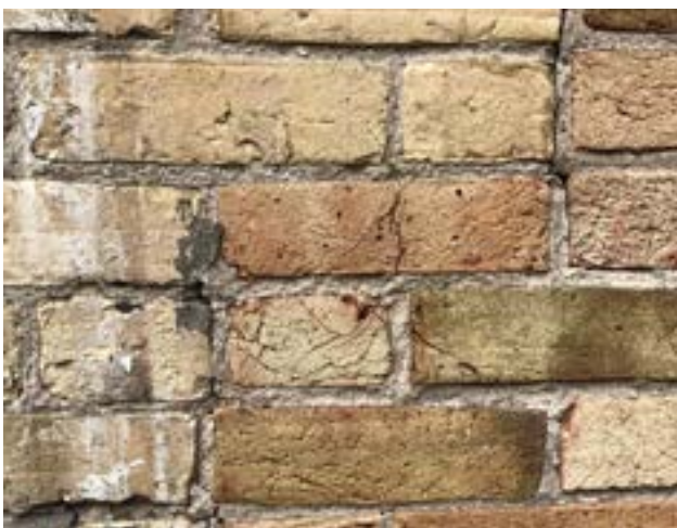
Figure. 2.6. Incompatible mortar & cracked brick
