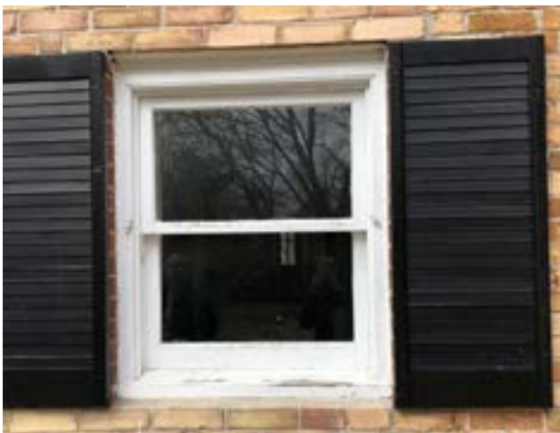
Figure. 2.38. Partially deteriorated original wooden windows with non-original shutters
