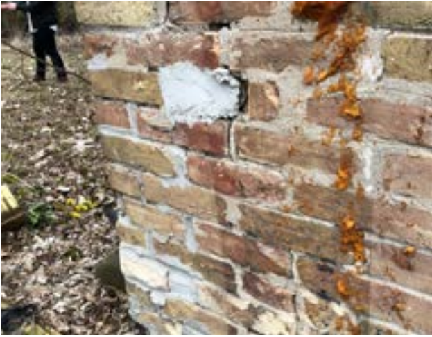
Figure. 2.10. Southwest corner brick in poor condition
