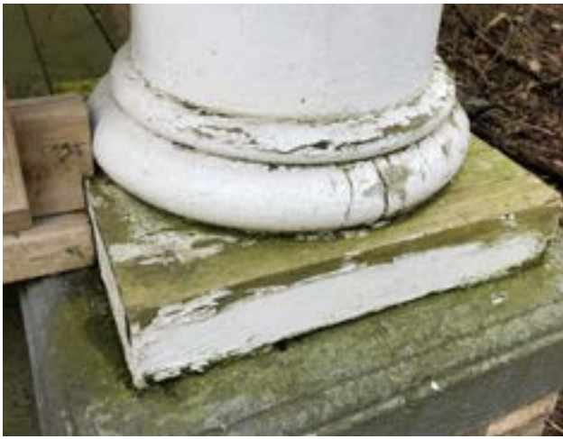
Figure. 2.36. Deteriorated original column bases at front porch
