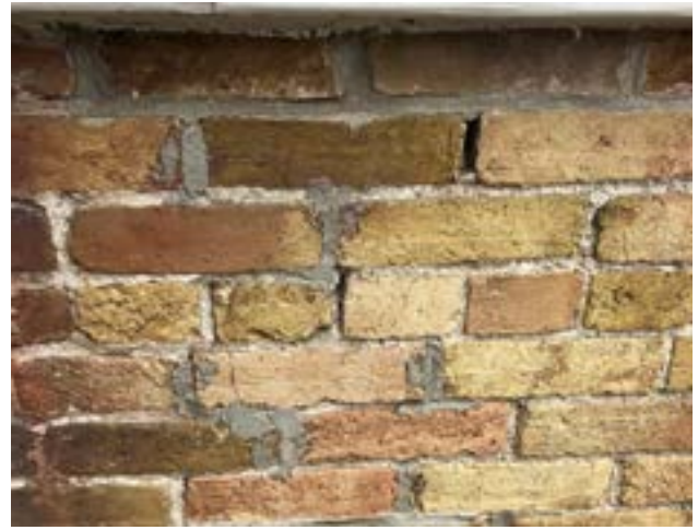
Figure. 3.20. Incompatible mortar to be removed
