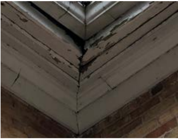
Figure. 2.31. Deteriorated original soffits and fascia
