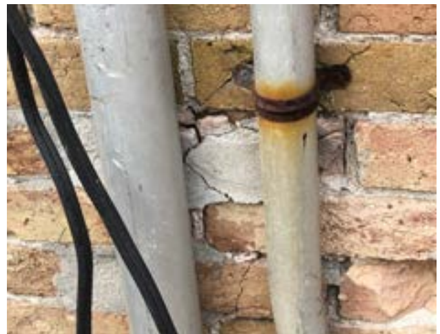
Figure. 3.22. Spalled & cracked brick to be removed & replaced
