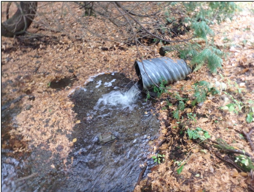
Photo 12: Photo showing the perched CSP and plunge pool at the pond outlet (Photo Date: Oct 22 nd , 2020).
